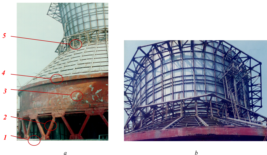
Figure 1. Large-sized cooling tower:
