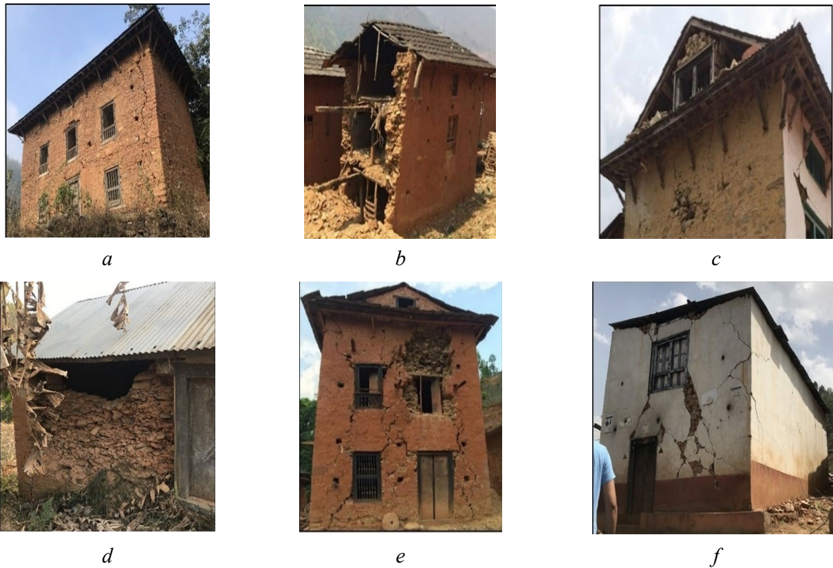
Figure 1. Failure mode in masonry building during earthquake: a — separation of short wall at cross section; b — complete collapse of short wall; c — collapse of gable wall; d — out of plane bulging; e — in plane damage with opening; f — shear damage
