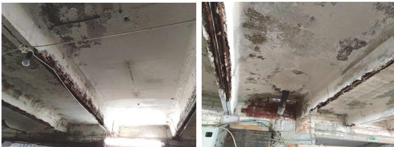
Figure 1. Corrosion damage to the coating of an industrial building in Moscow
