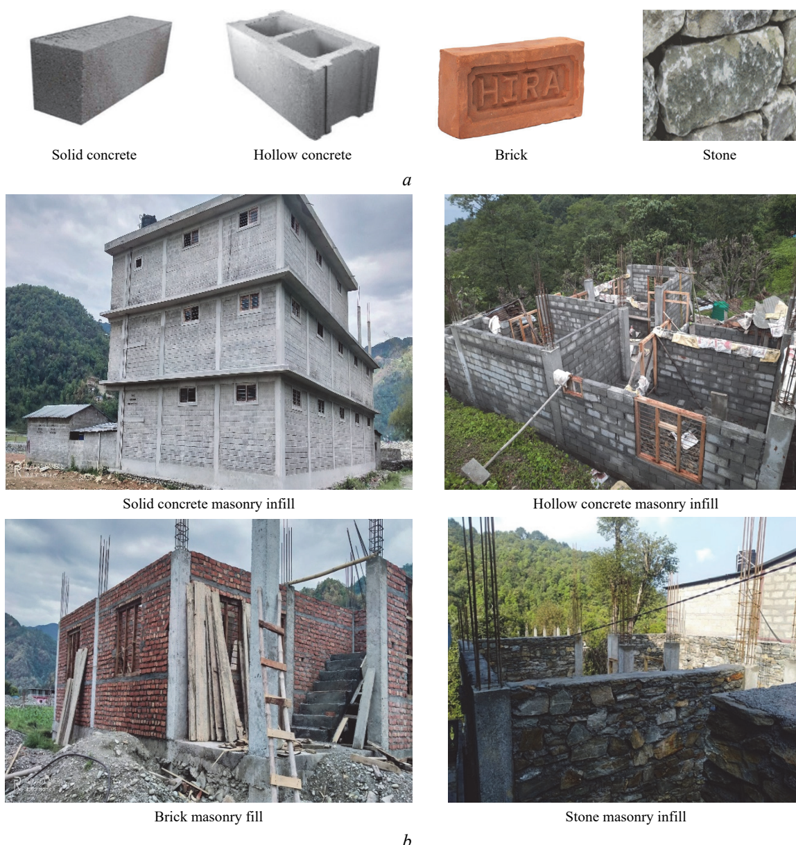
Figure 2. RC building construction trends: a – masonry unit; b – structures with masonry infills
