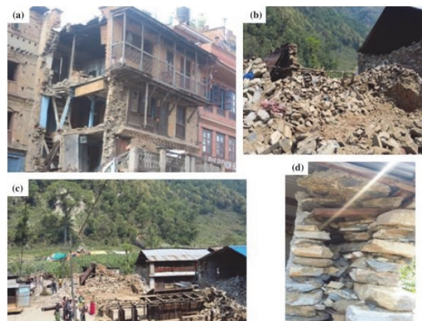
Figure 2. Failure mode of masonry houses:
