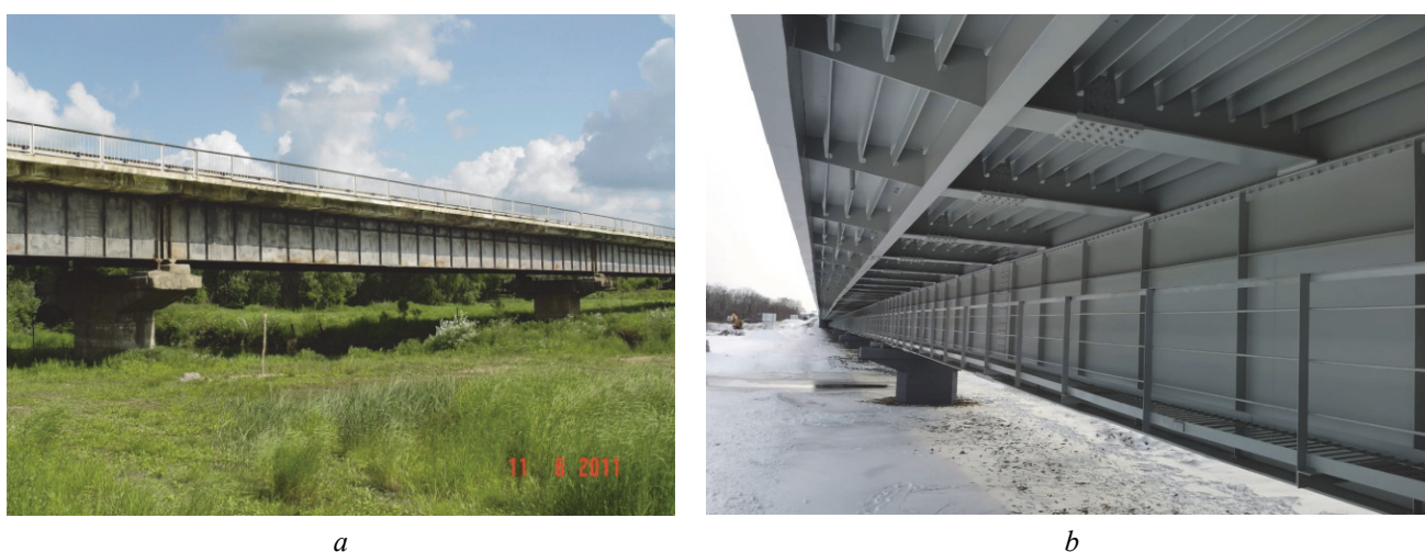
Figure 2. Side view of the span structure of the bridge across the Kabarga river: a – before overhaul; b – after overhaul, 2020
