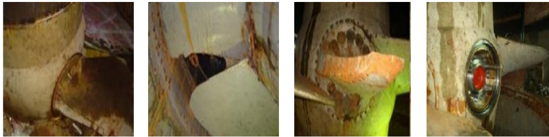
Figure 8. Damaged runner blades of the Haditha HPP Kaplan turbine: image courtesy of the Ministry of Electricity, Iraq Source : photo by the authors
