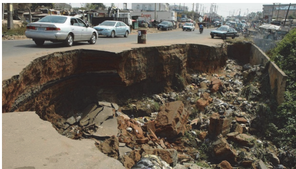
Figure 2. Soil erosion in Abia state
